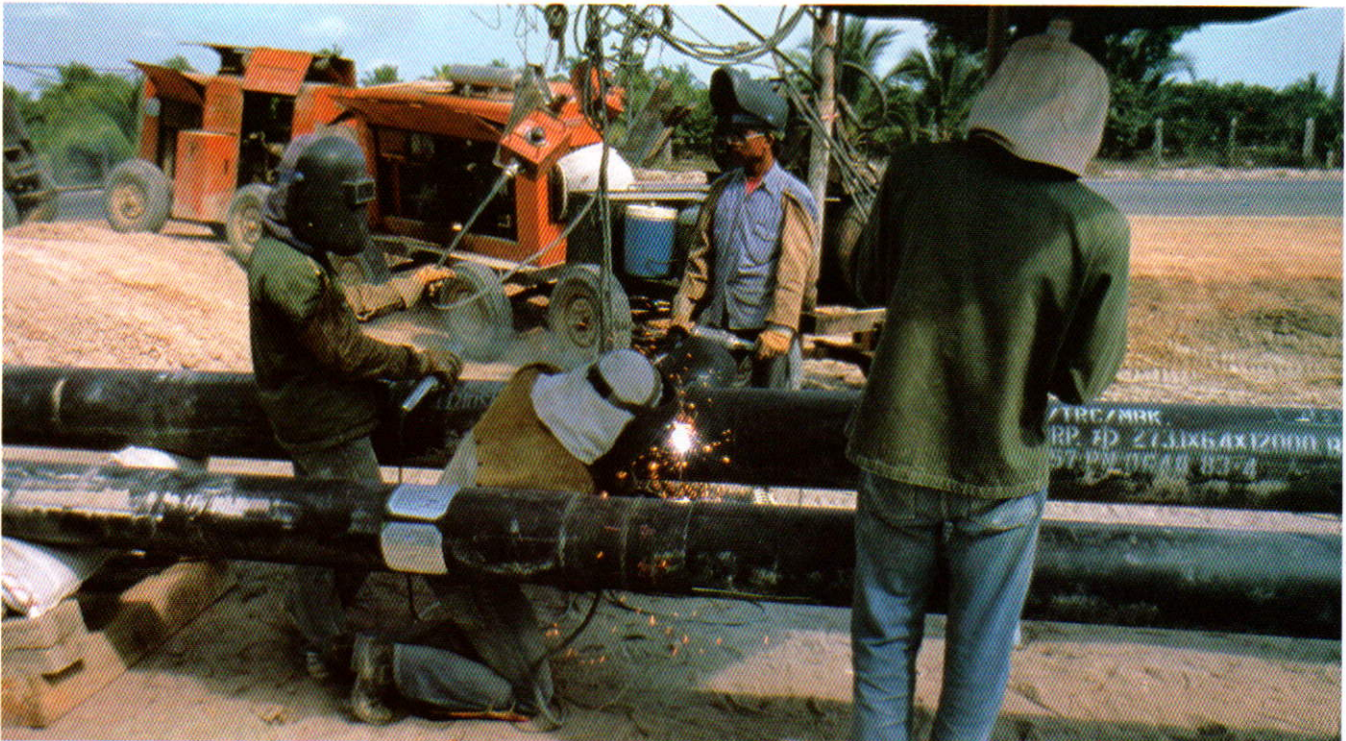
1. Product pipeline from gas separation plant to marine terminal storage tank.
