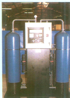
Water & Waste Water Equipment
