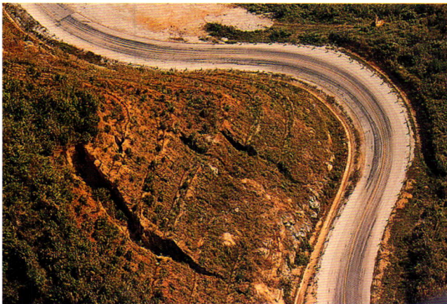
Land slippage caused by road construction.
