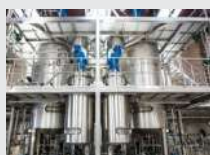
Biorefinery Pilot Plant (2563-2565)
