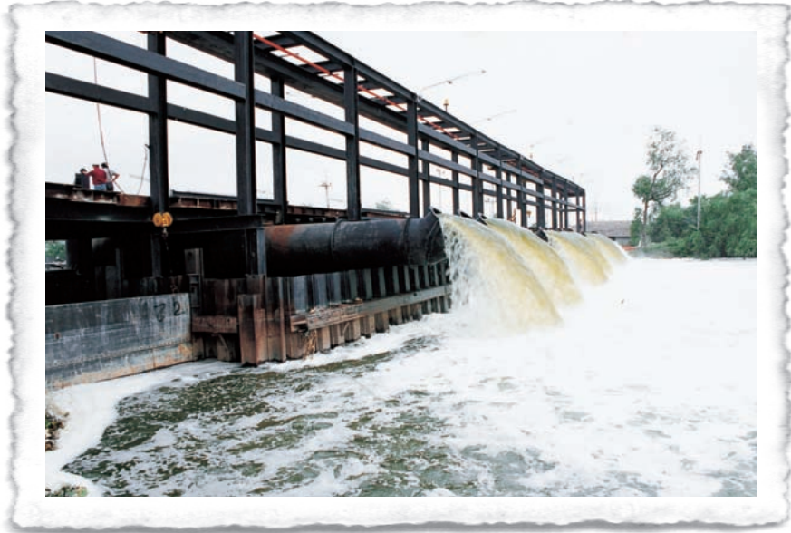
The Mahachai water gate and pumping station.
