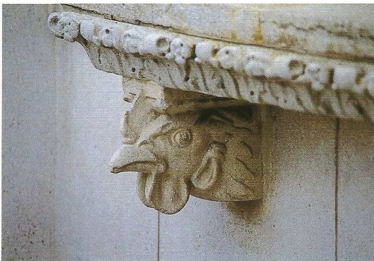
The rooster head decorations are found all over the building underneath the windows, at the end of the rainwater drains and of the balcony's supporting beams.
